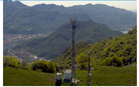
Routers, servers, data centers, base station cooling, mobile communications
