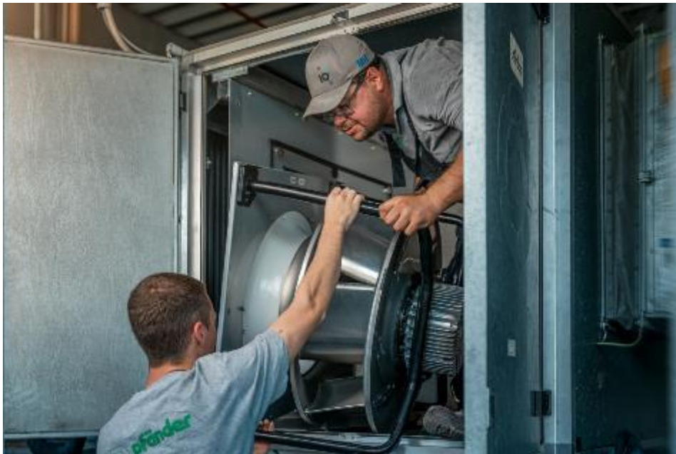
Figure 2: In many systems, EC fans were replaced with the latest generation of EC fans.
