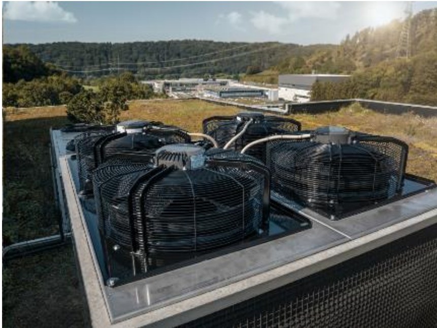
Figure 1: For the retrofit at ebm-papst, a total of 161 systems with fans suitable for replacement were identified. This picture is from Mulfingen.
