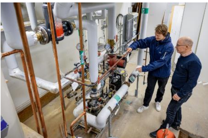
Image 2: The retrofit project in Gyllenstiernsgatan was just the beginning: Stockholm Exergi and ebm-papst are planning to make other buildings in Stockholm more energy efficient.
