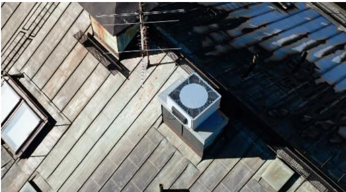
Image 1 a + b: Data from the ventilation system can be viewed and analyzed live via the cloud.
